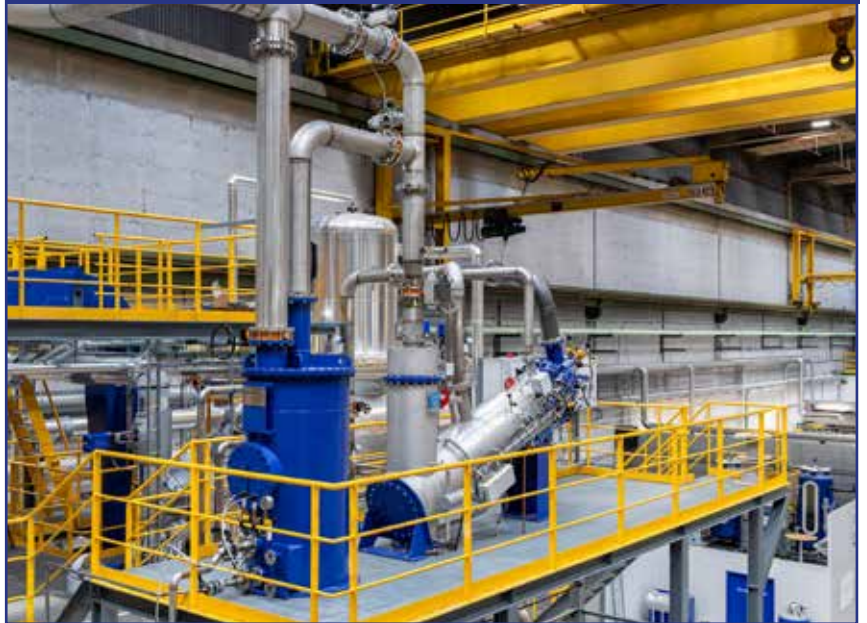
The Alfa Laval Smit inert gas system in Alfa Laval Test and Training Centre
