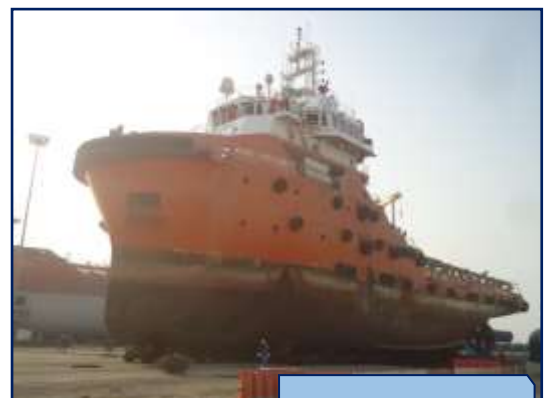
BEFORE THE REPAIR
